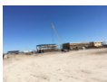
Construction of restrooms and locker rooms with east side stands and pavilion
