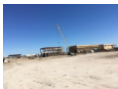
Construction of restrooms and locker rooms with east side stands and pavilion
