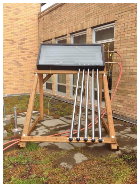
Figure 7. Hybrid solar collector on green roof [4].
