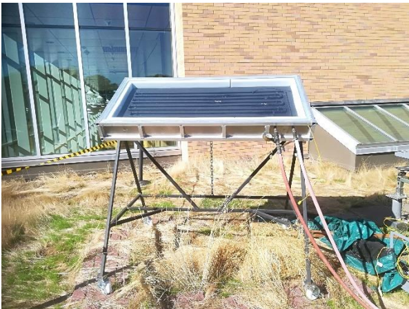
Figure 8. Flat plate solar collector on green roof.
