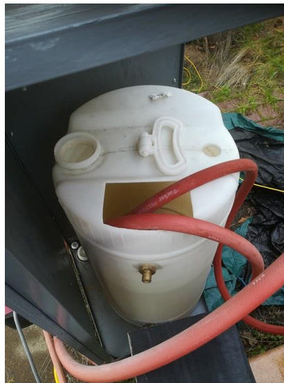
Figure 18. Plastic tank and connection tubes of the system.
