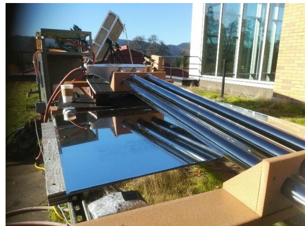
Figure 20. Upgraded evacuated tubes with mirrors underneath and the tilted flat plate collector in the background.
