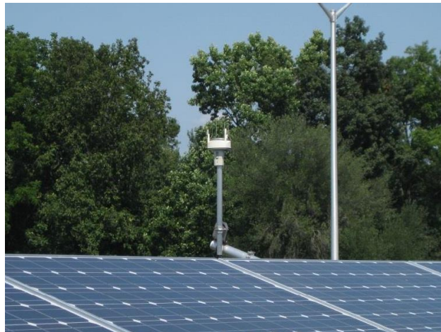
Figure 30 Wind sensor at the ground array (Boyd, 2015)
