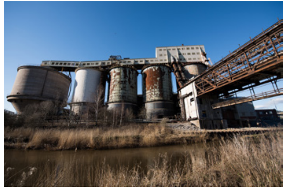
Fig. 35: Corroding metal on the silos of an abandoned factory.
