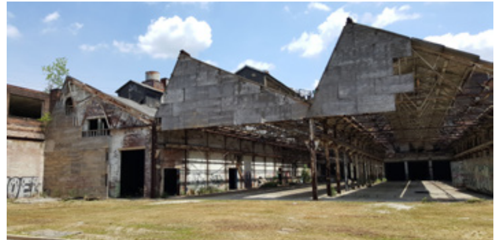
Fig. 55: The steel structure of the former assembly hall seen from the outside (from western direction). The aisle on the very left shows brick walls on the inside that were later induced.
