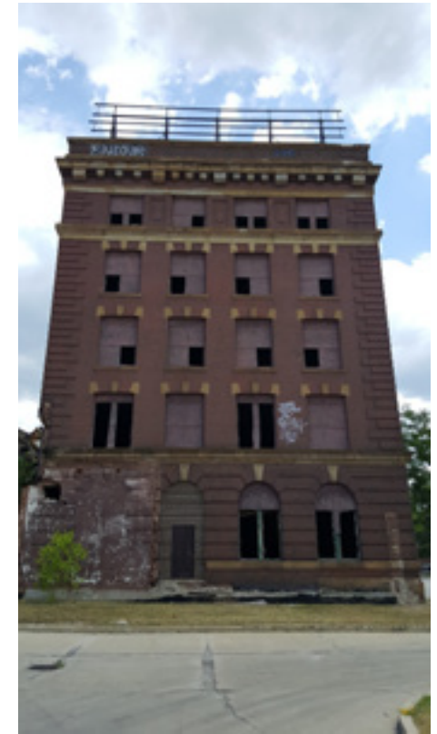
Fig. 60: Damages in the brickwork of the western face of the main building.
