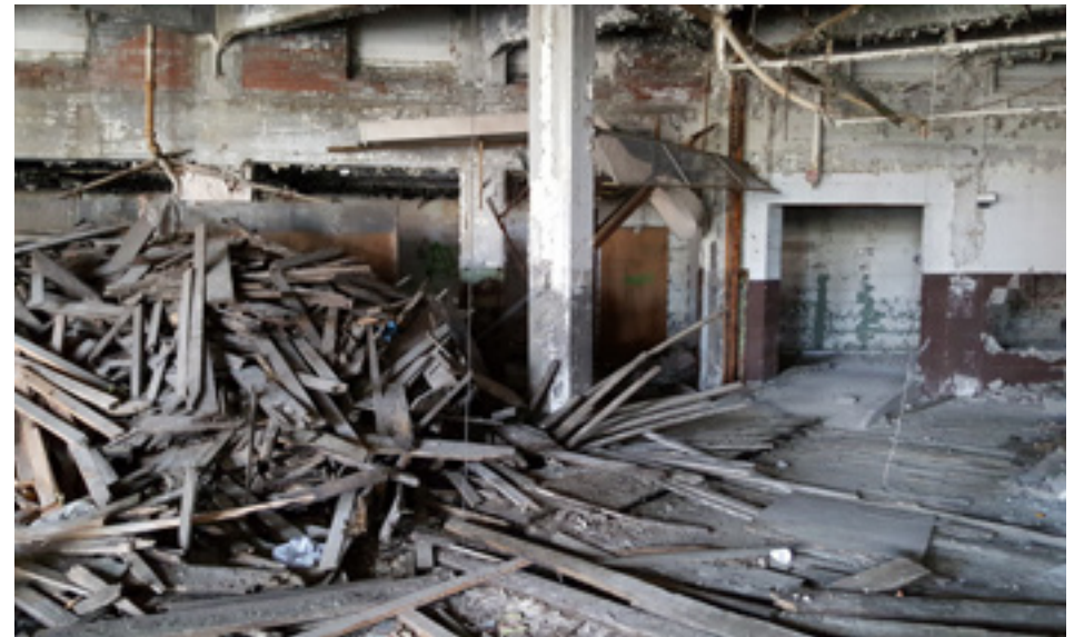
Fig. 62: Debris of former fitout.
