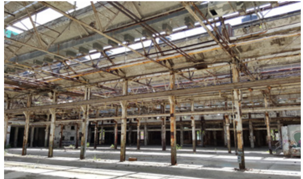
Fig. 61: Corrosion of the steel structure in the assembly hall.
