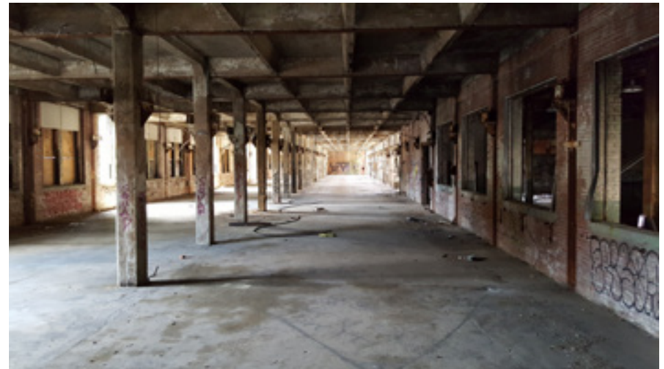
Fig. 58: Inside the main building on ground floor level, showing the open structure.
