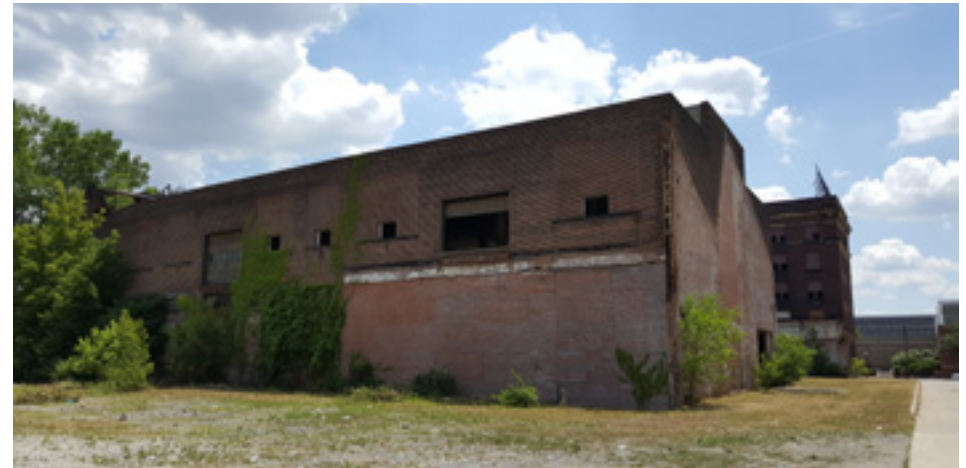
Fig. 52: The north facade of north building indicating a former addition to the complex that has gotten removed.
