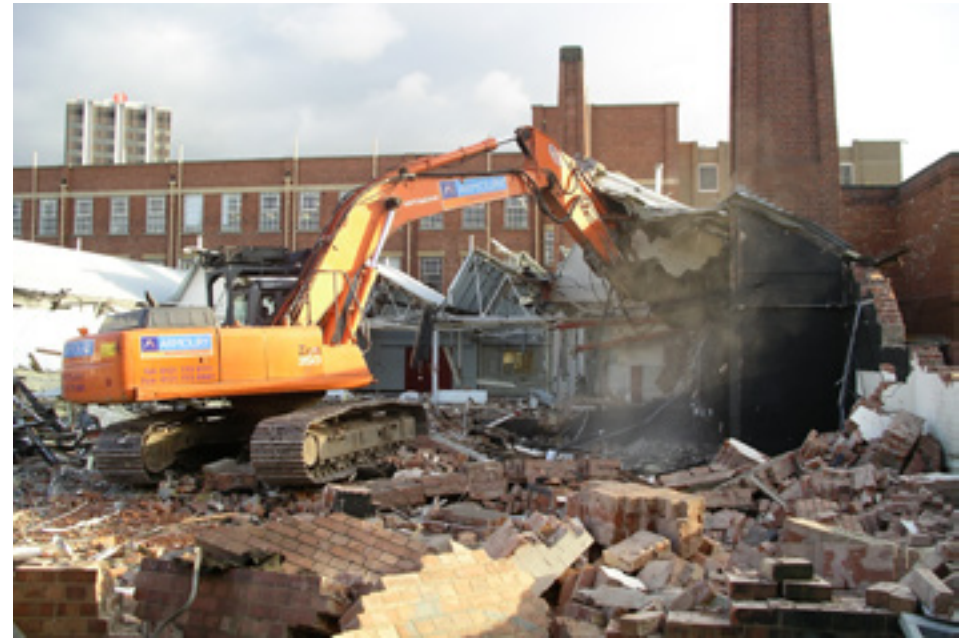
Fig. 16: Demolition of an industrial building in Coventry (England). The existent value of the brickwork which would be expensive to create nowadays is lost.
