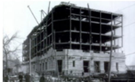
Fig. 24: The steel skeleton structure of a railway station in Scranton (Pennsylvania, United States) being clad with a limestone facade in 1907.
