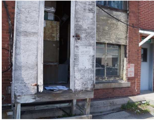
Figure 33: On-site visit, altered opening
