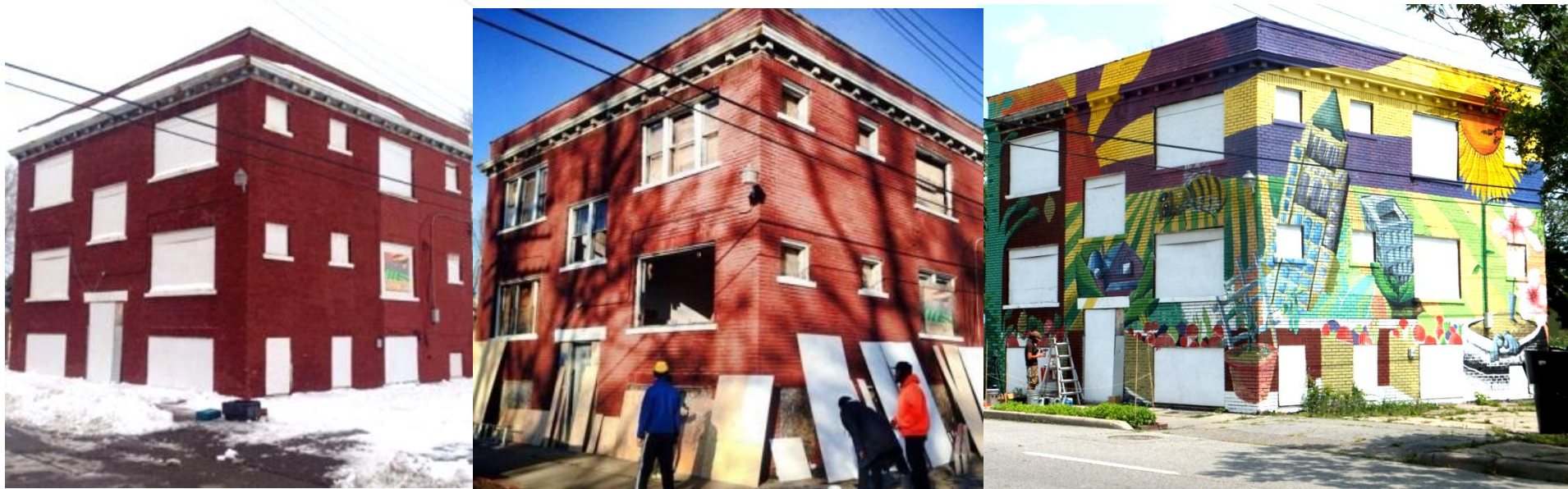
Figure 20 Photo series of the future community center, work in progress Photo 1 and 2 ( https://www.crowdrise.com/windowsformufi/fundraiser/MUFI ) Photo 3 (Photographed by Andrea Korber, 2014)
