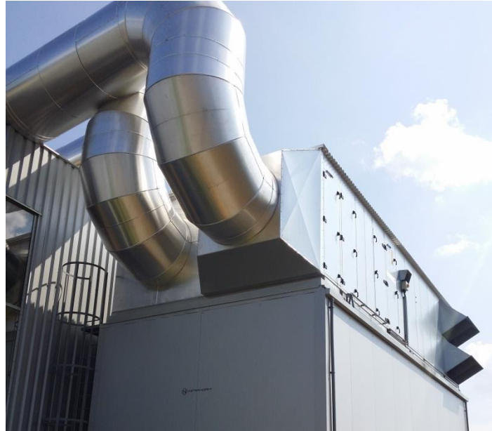
Figure 22: Heat recovery system MAGNA STEYR Fuel Tec Sinabelkirchen [cf. 74]
