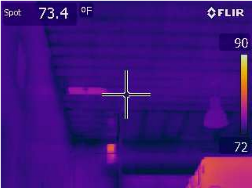
Figure 48: IR picture of garage ceiling, Fire Station 11, 11.10.2012
