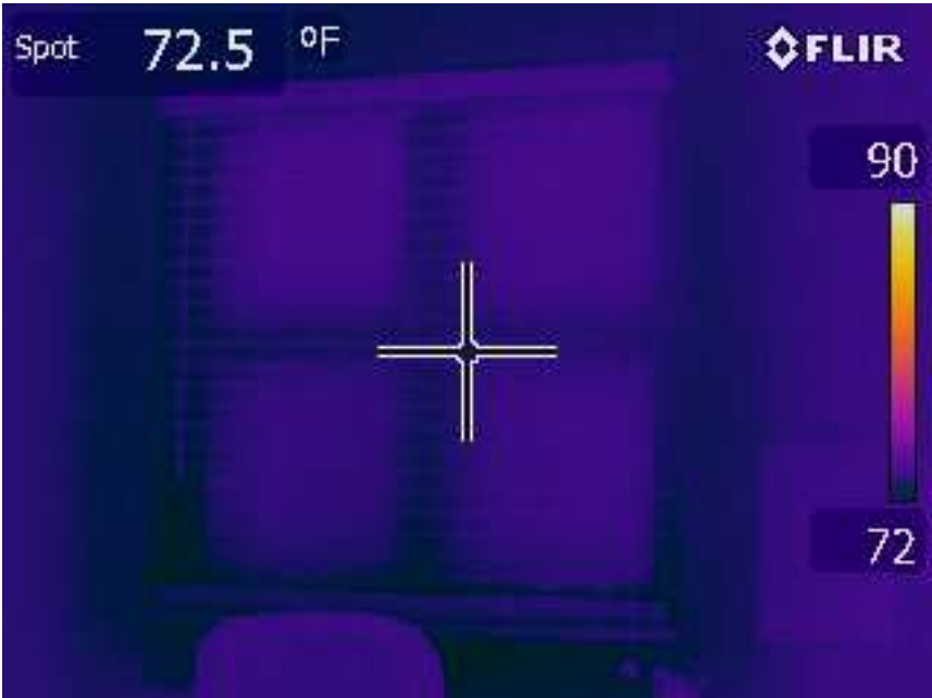
Figure 49: IR picture of insulated window, Fire Station 11, 11.10.2012
