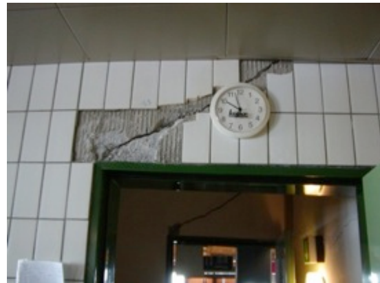
Fig.58: Deformation of old restaurant.
