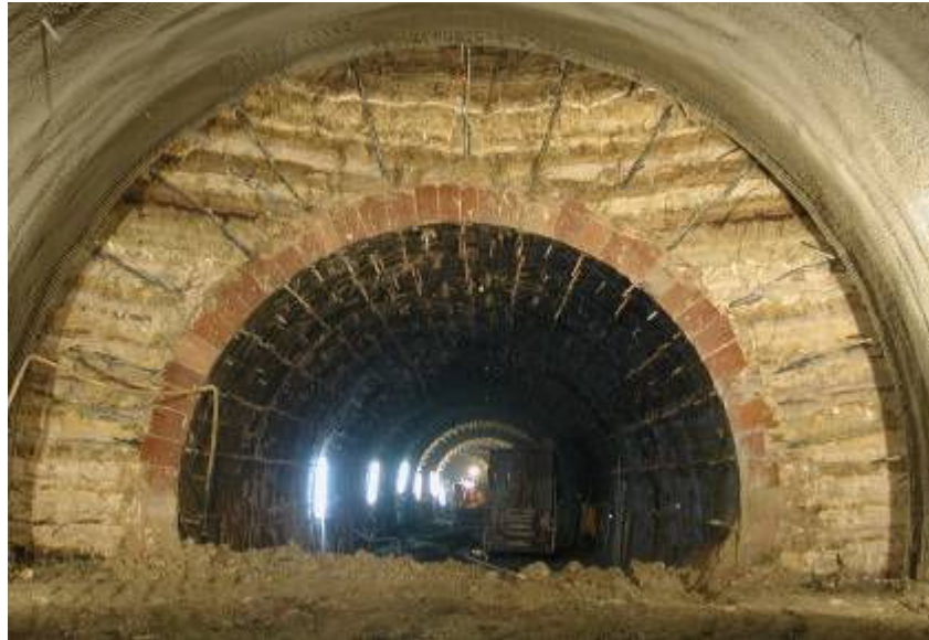
Figure 2: Photography of tunnel face with the different layers (source Beton- und Monierbau)
