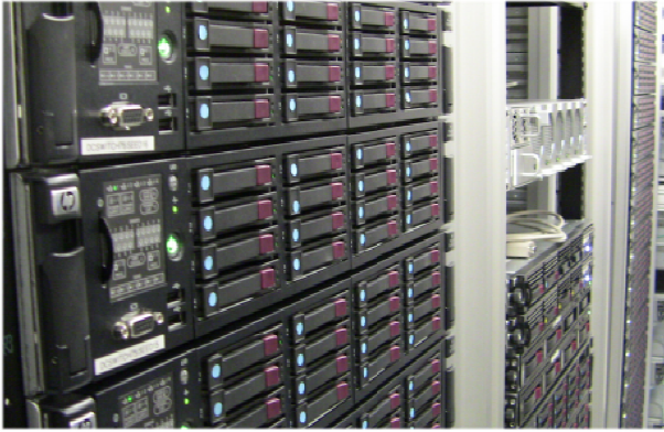
Figure 7 - Test bed hardware
